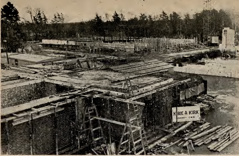
Facing east: showing the concrete work on the ground floor and several of the brick partitions
